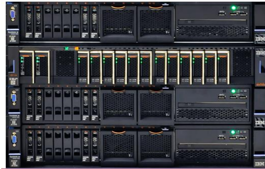
Figure 25 IBM FlashSystem A9000 Storage Front View
