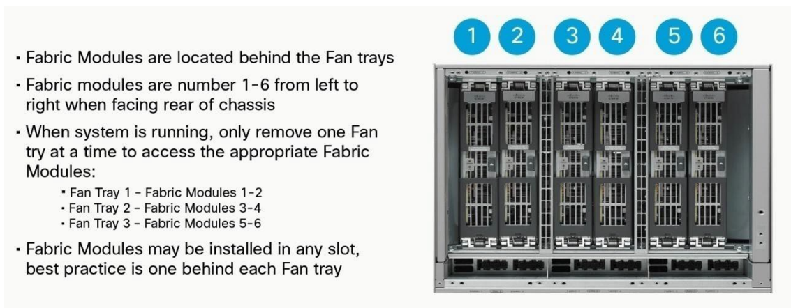
Figure 11. Back of a Cisco MDS 9706 Chassis with Its Six Crossbar Fabric Modules Exposed
